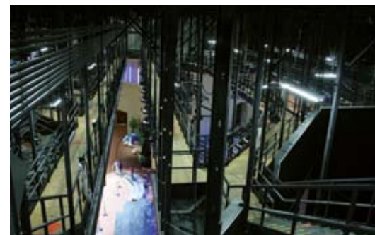
An extensive catwalk system enables Idlewild's lighting technicians to access all architectural and theatrical lighting fixtures in the facility. A large elevator provides access to the catwalks from the loading dock, greatly facilitating the use of rental gear and the maintenance of installed equipment.
